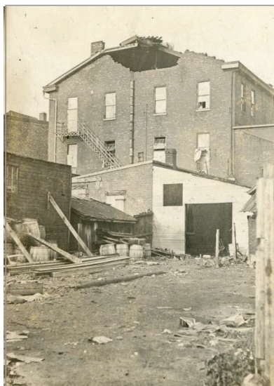
A photo featuring tornado damage to the rear of the Mart Miller building on North Sandusky Street. Circa 1912.
